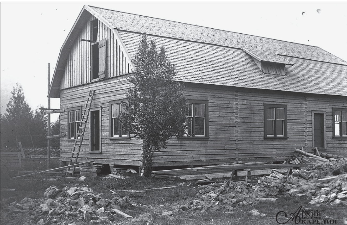
Dining room, kitchen and bakery during the construction (Courtesy of the National Archive of the Republic of Karelia).
