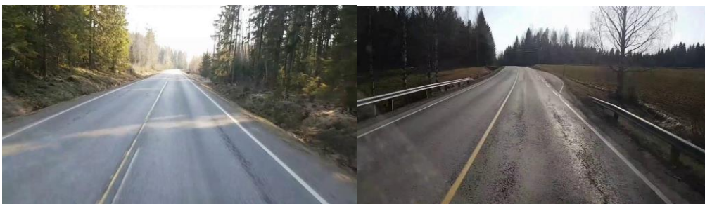
Figure 13. Person 1: severe crack. Computer vision: no crack identified (2 instances).
