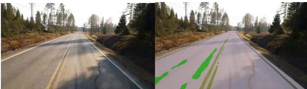
Figure 16. Computer vision: severe crack. Person 1: no crack detected (2 instances, marked in brown in the segmentation image).
